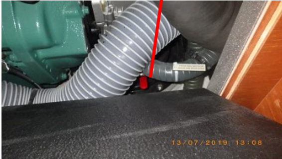
Engine cooling water inlet
