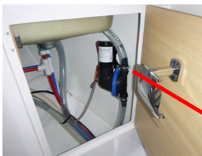
Shower pump switch
