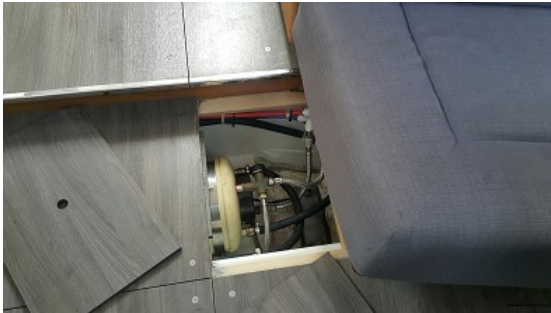
Water heating switch
