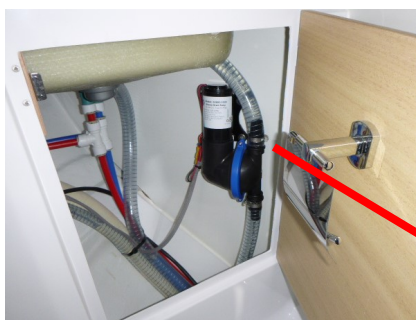
Shower pump switch
