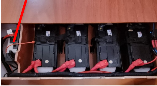
Battery charger / 4 x service batteries
