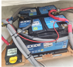
Bowthruster batteries in bow locker under plastic hatch
