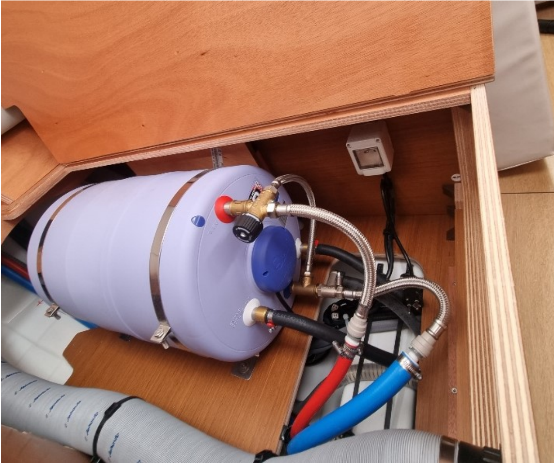
Water boiler/heater is located under the seats in saloon.
