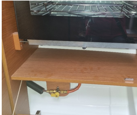
Gas valve under the stove
