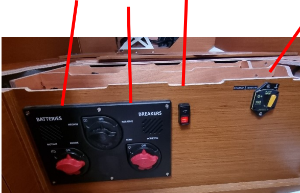
Switches of Servis Start Bowthruster baterries and anchor
