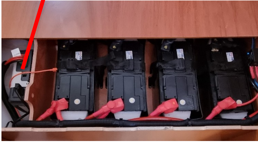
Battery charger / 4 x service batteries
