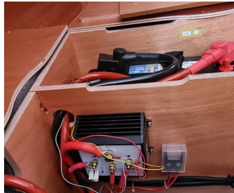
Starter batteri, instrument fuses ,isolator are located under the bed in aft port cabin
