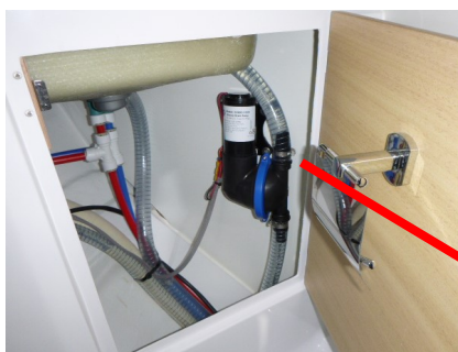
Shower pump switch
