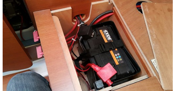
Engine battery located under the bed in port aft cabin.
