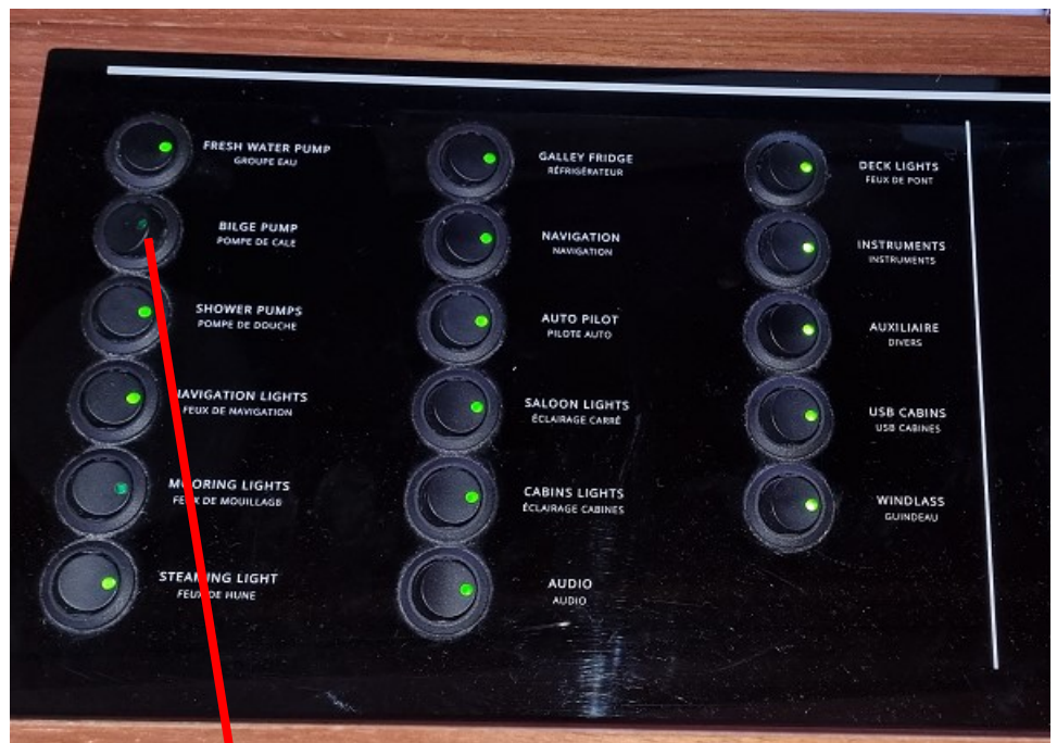
Bilge pump switch
