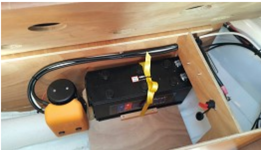
Bowthruster battery under the bed of bow cabin
