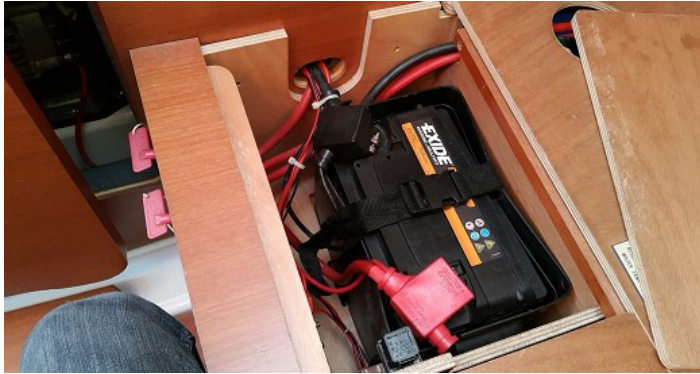
The engine battery, main service and start breakers with red key are located on the wall of port aft cabin .
