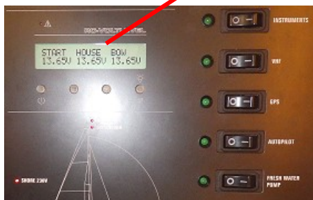
Fresh water pump switch.
