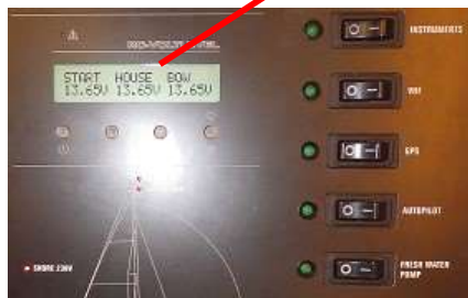
Fresh water pump switch.
